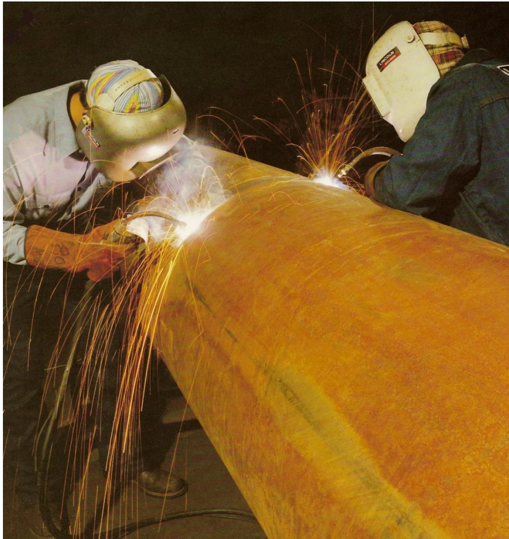
Two welders performing arc welding on pipe - requires full-time attention of workers (photo courtesy of Lincoln Electric Co.)
